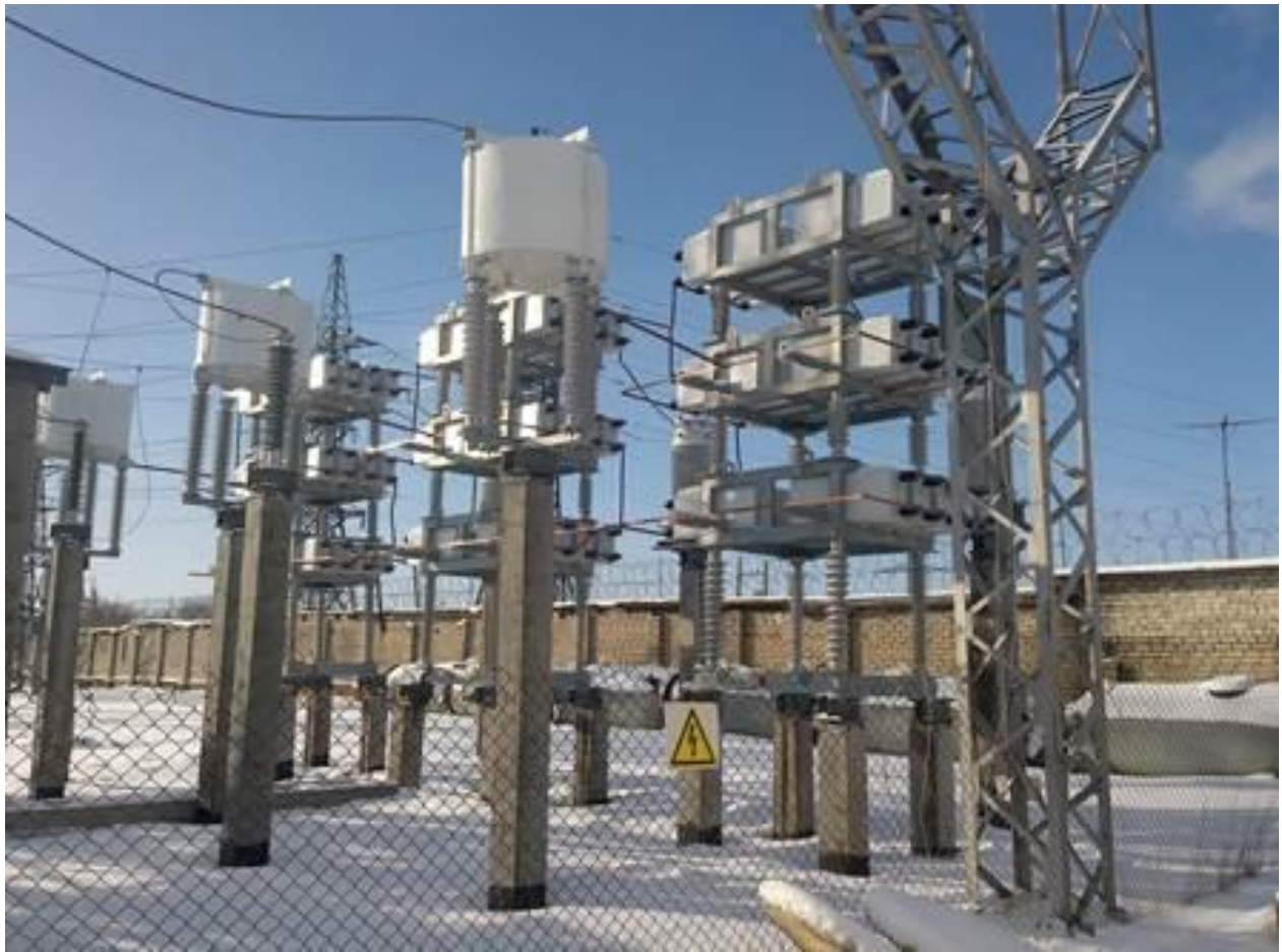
Photo of a 110 kV capacitor bank at Efremov SS (Tulenergo)
